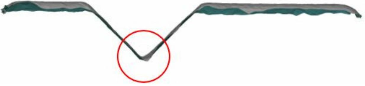
Figure 4.7: The shape of the scanned point cloud representing the defect after meshing the points.
